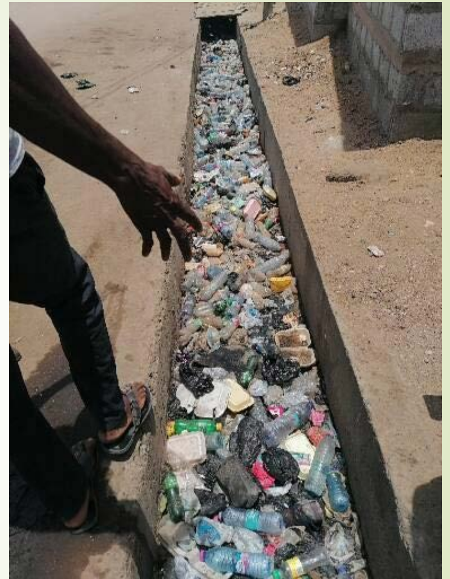
Gutters are filled with plastics close to food joint
